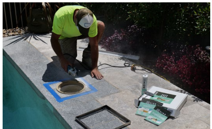
This retrofit took about 90 minutes. It all depends on the material to cut out and skill of the operator.
